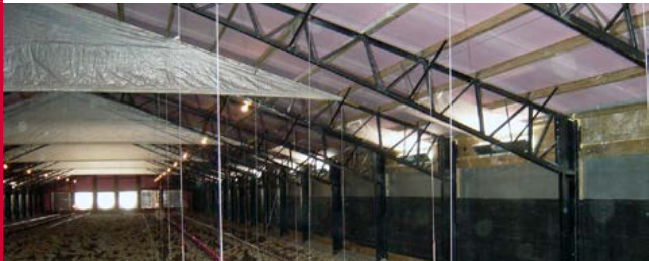
Figure 6.19 Example of air deflector/baffle placement in a tunnel-ventilated house.
