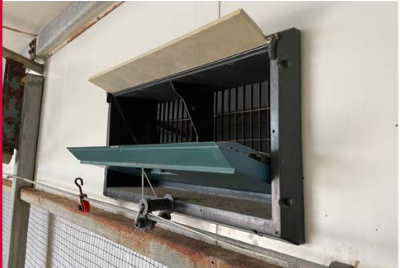
Figure 6.10 Example of a good-quality air inlet.
