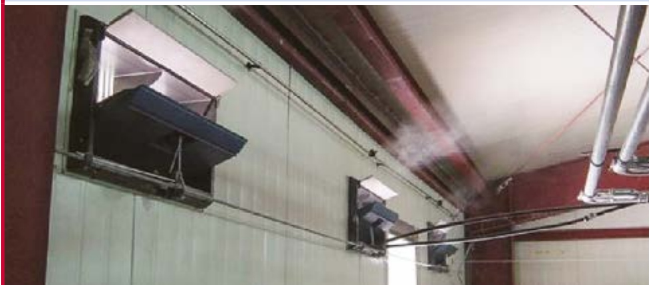
Figure 6.25 Example fogging system for a cross-ventilated house.
